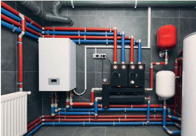
Domestic heating system room
