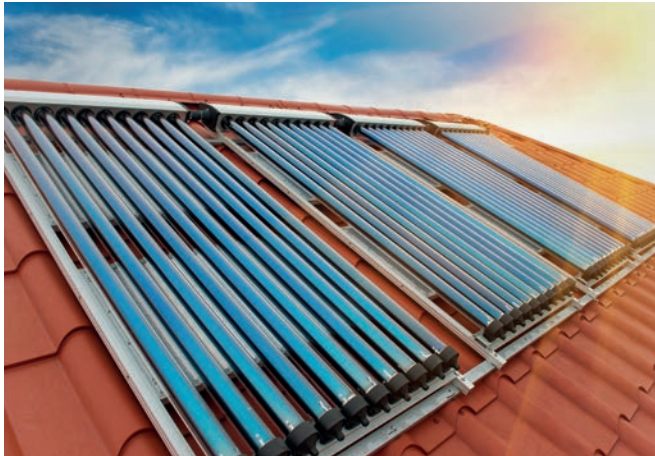
Thermal solar panels for water heating
