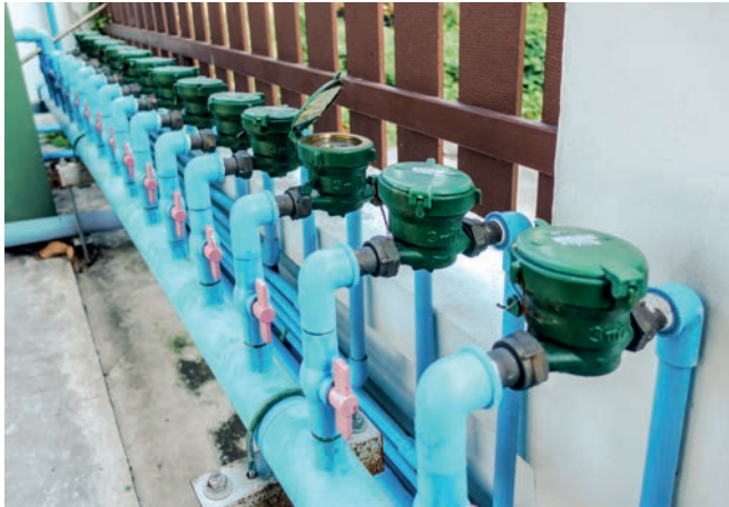
Water meter and water pipe system
